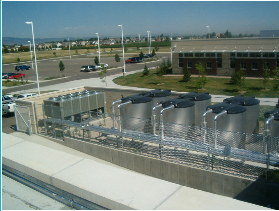
Ice Storage Tanks and Air-Cooled Chiller
