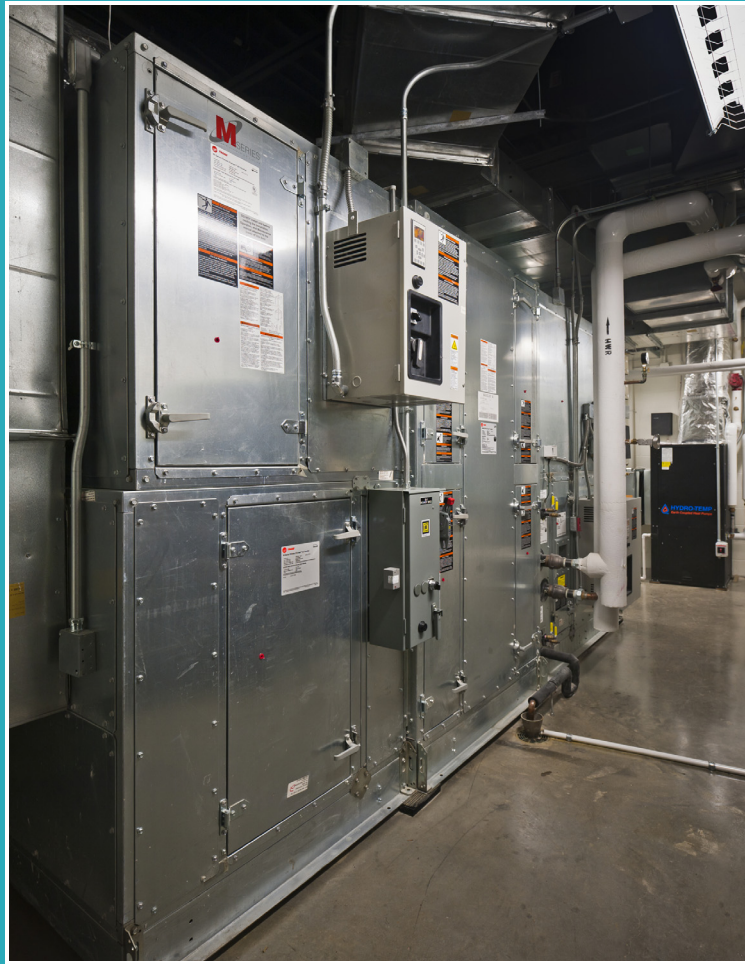
Outdoor Air-Handling Units
